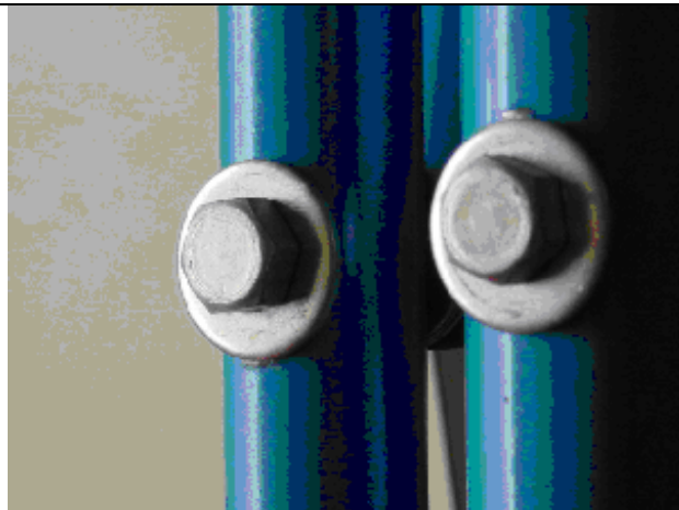
Not Correct Washers and Bolts Head 1
