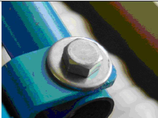
Not Correct Bolts Head 3
